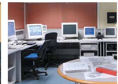
The entire plant is monitored and controlled remotely.
